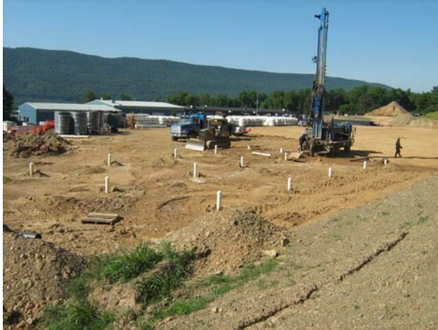
Geo-Thermal Well Field
