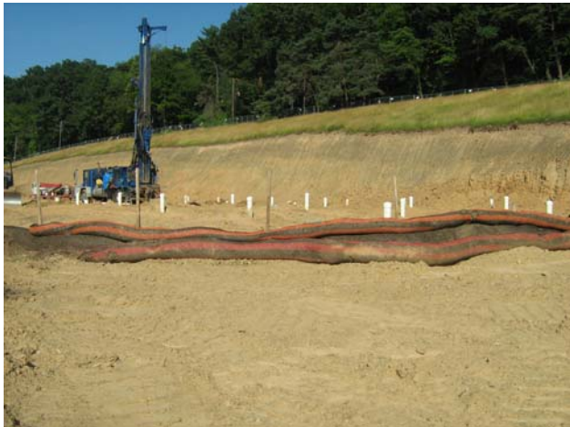
Geo-Thermal Well Field
