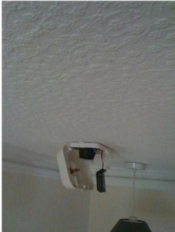
battery to be replaced
