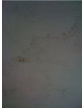
around 2 feet square, possible leak, to investigate
